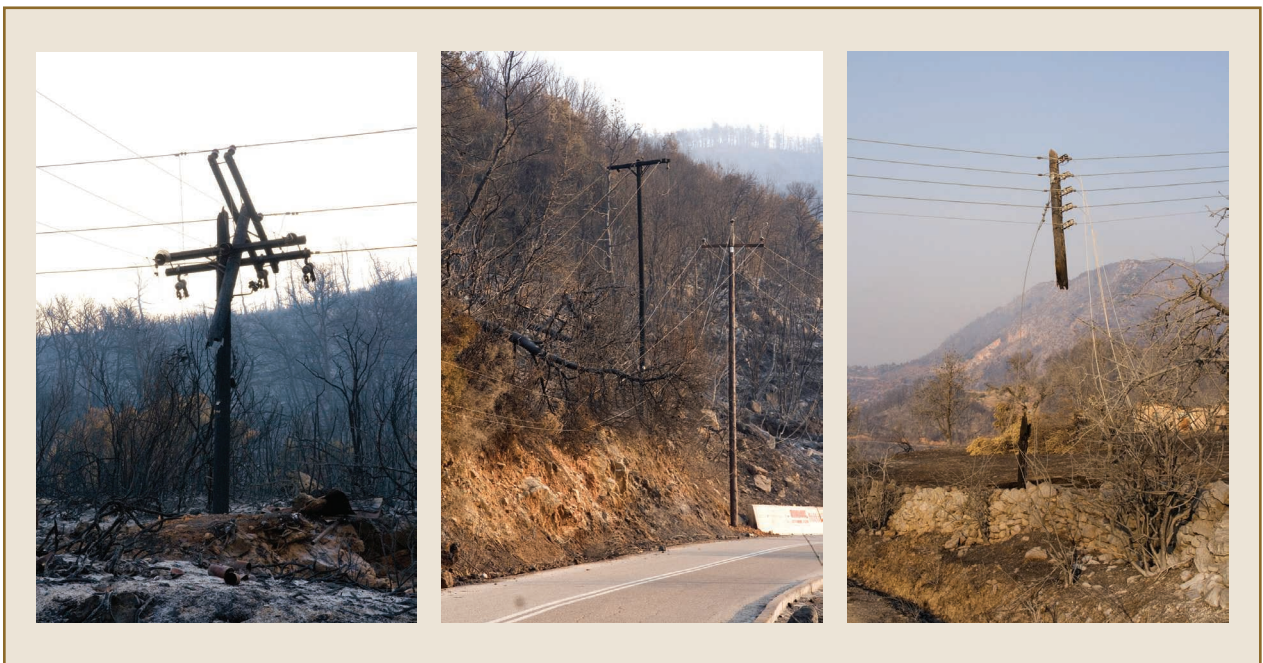
figure 5. Damaged lines and poles from the 2007 forest fires in Greece. (Source: Courtesy of Public Power Corporation, Greece.)
